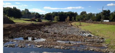
Above: hydraulic model, MMSK students observing construction, U.of L. research cells, built channel.
